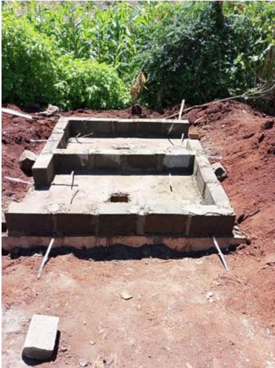
When the cement slab was "cured" we added the base for the walls.
