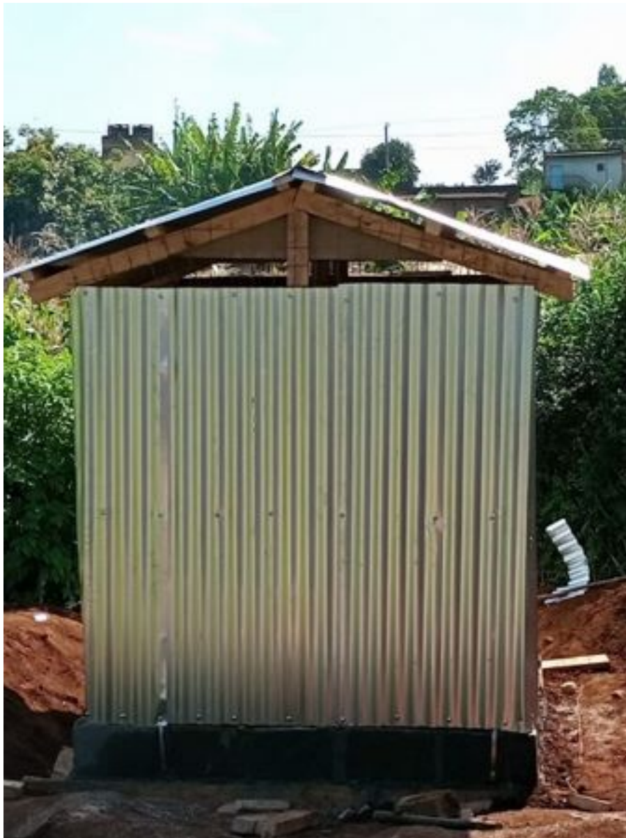
Finished. Now we need to extend the sidewalk to the new toilet building.
